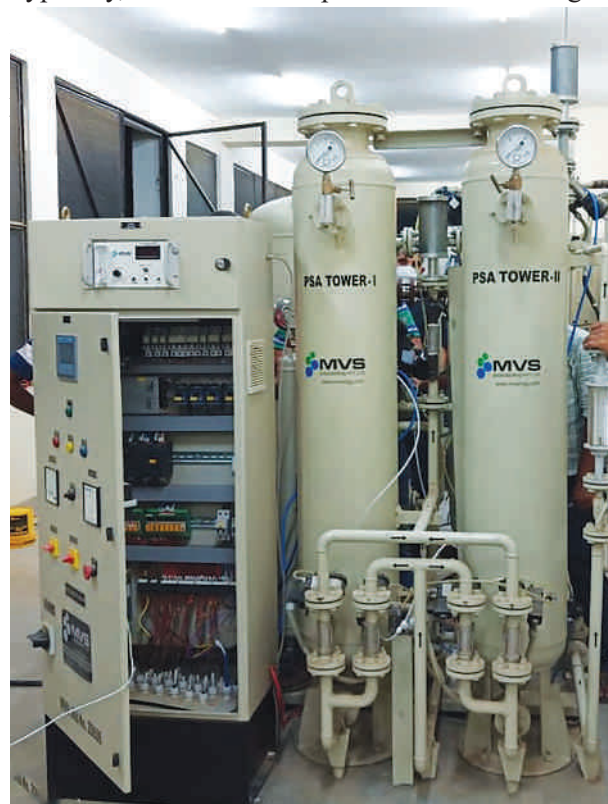
The PSA-based oxygen generator developed at CSIR-CEERI, Pilani
