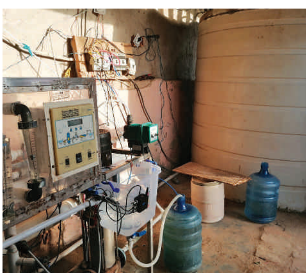
Installed Device at a nearby water purification plant
