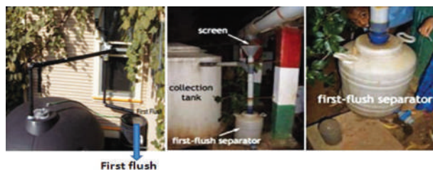
Installed rainwater harvesting system
