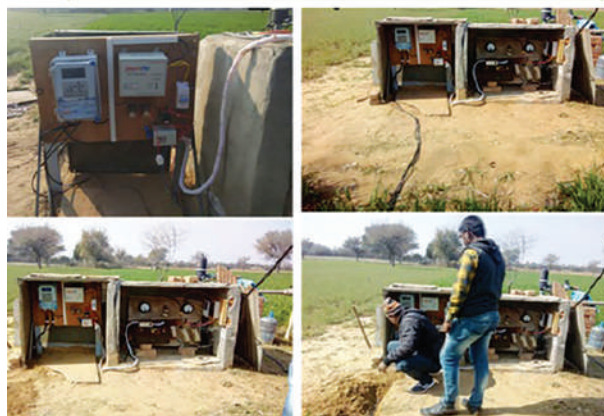
General layout and field installation of the three-phase controller system
