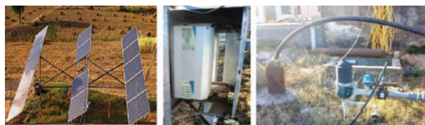
Field-installed PV solar panels (235W), Lorentz PS4000 controller and submersible pump
