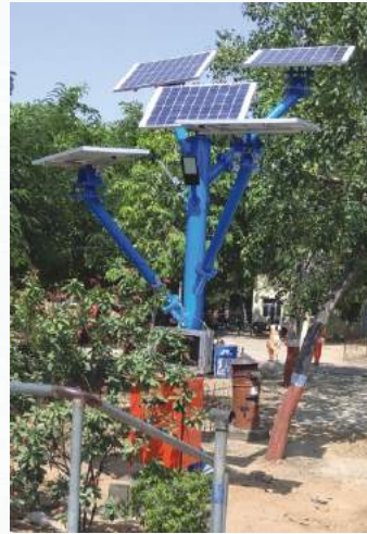
500 W solar tree installed at CSIR-CEERI
