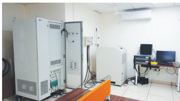
Actual grid-tied inverter test setup at CSIR-CEERI's IIIH, Jaipur Centre
